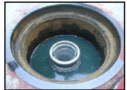
Spill bucket that contains liquid
