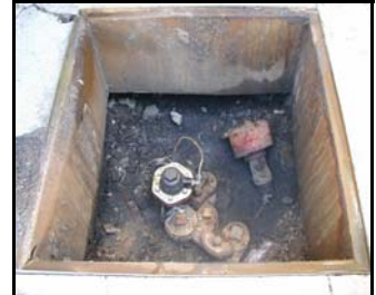
Uncontained turbine sump
