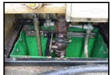
Contained dispenser sump
