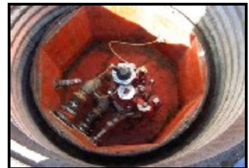
Contained turbine sump
