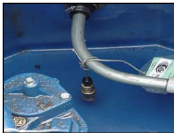
Liquid sump sensor
