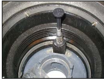
Spill bucket drain valve
