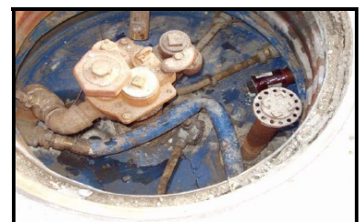
Flexible piping is kinked
