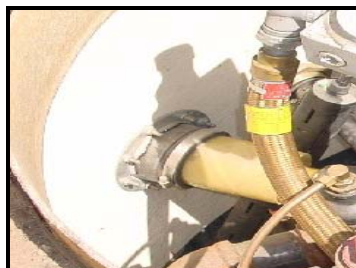
Sump penetration seals in good condition
