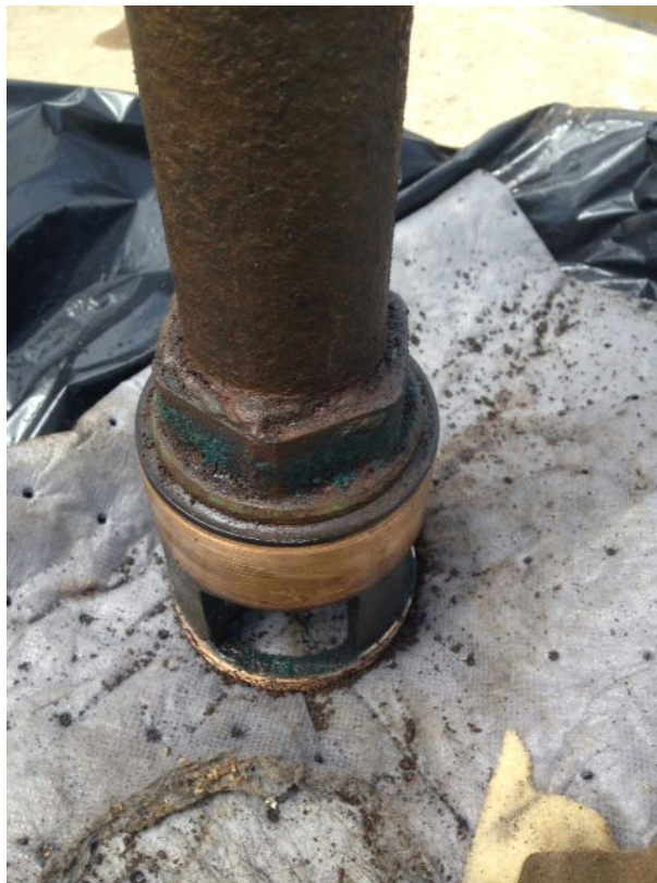
Figure 2: The suction tube column. This is the upper length of the pipe. Note the blue discoloration of brass (indicative of exposure to acid). This photograph was taken after removal of 1/8" to 1/4" thick precipitated material.
