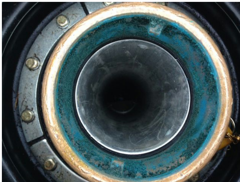
Figure 4 : Brass fill port at DPS #2. The blue-green precipitate is the result of an oxidation-reduction reaction in the system
